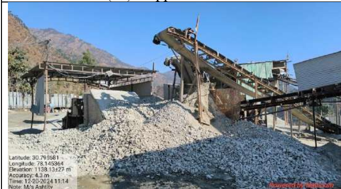
Pic. (05) Transfer point of the Grit
